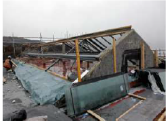
Looking (facing Mackinlay St): new steelwork to the roof light (NB: temporary waterproof protection partially removed).
